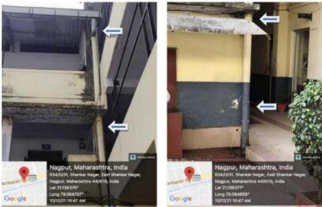
Pipeline of Water Harvesting System
