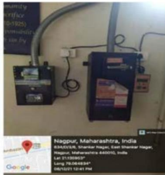
Incinerator machine in Girl's Common Room
