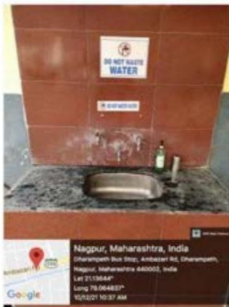
Taps to be replaced by Push Buttons / Faucets
