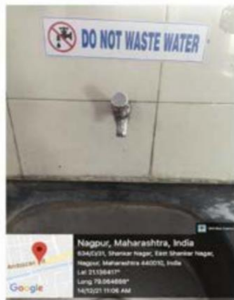
Push button taps installed at some points
